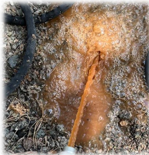
Flush of water tank
